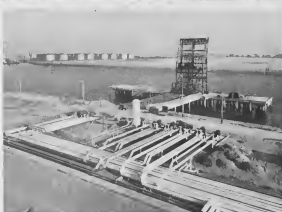
TWO PIERS were built to accommodate 50,000 deadweight-ton tankers in the western and southern legs of the harbor, above. Drain water, below, is subjected to special purification processes.
